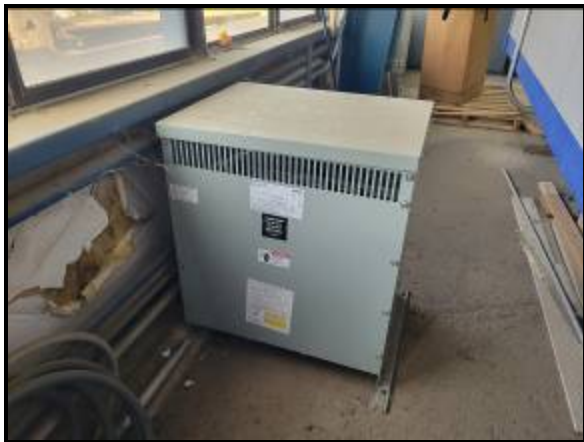
Existing 75 KVA Transformer Serving Panel "L-104"
