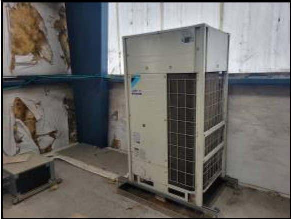
Existing VRF Heat Pump Serving Existing Driving Simulation Lab
