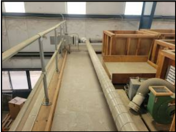
Existing Exhaust Fan & Ductwork Serving Existing Driving Simulation Lab
