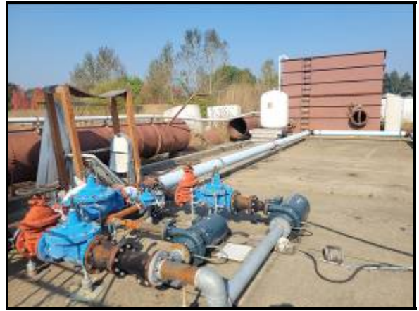
Existing Piping and Pumps to be Removed at Exterior Test Slab Area. Existing Above Ground Storage Tank Can be Seen.
