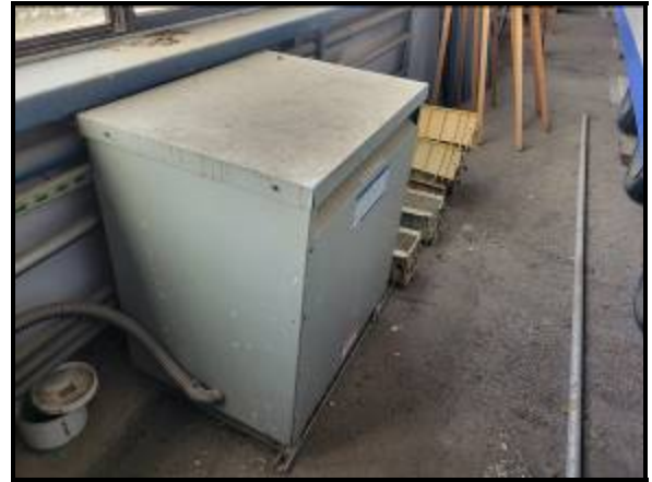
Existing 75 KVA Transformer in Area of Work for New Driving Simulation Lab Expansion
