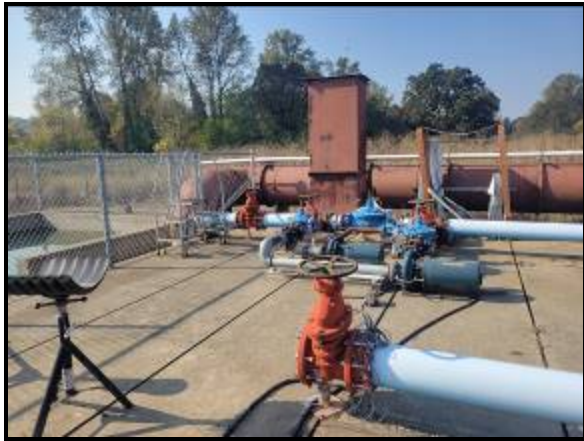
Existing Piping and Pumps to be Removed at Exterior Test Slab Area
