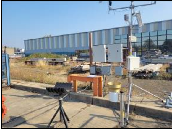
Existing Electrical Panels at Exterior Test Slab Area
