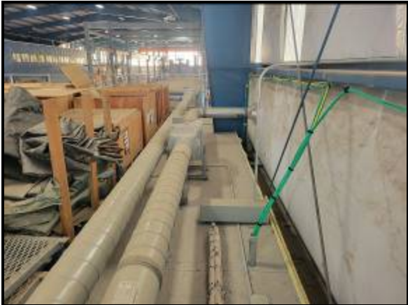
Existing Ventilation Fan & Ductwork Serving Existing Driving Simulation Lab
