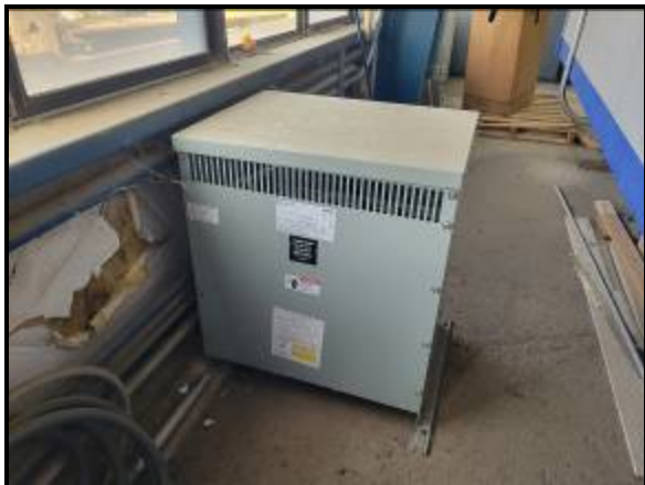
Existing 75 KVA Transformer Serving Panel "L-104"
