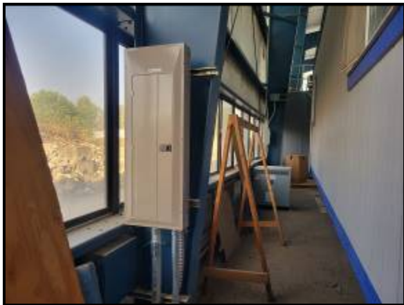
Existing Electrical Panel "5X"
