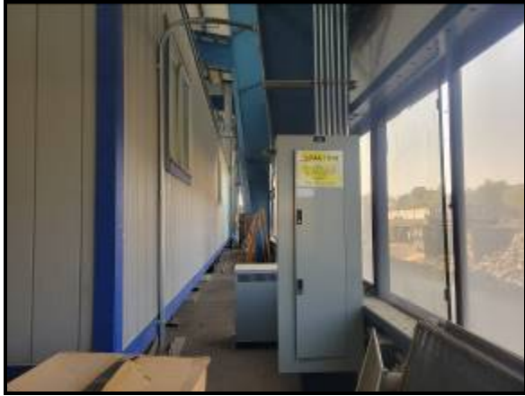
Existing Electrical Panel "L-104" Serving Existing Driving Simulation Lab
