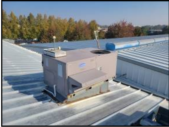
Existing Carrier Heat Pump Rooftop Unit Serving Second Floor Area on East Side of West Wing
