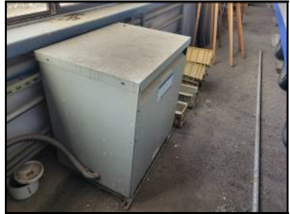
Existing 75 KVA Transformer in Area of Work for New Driving Simulation Lab Expansion
