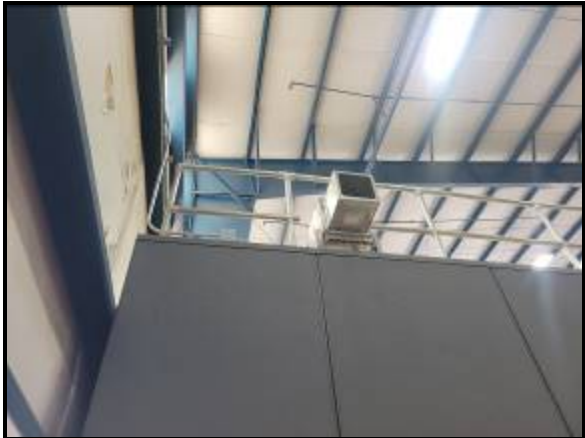
Existing Exhaust Fan Existing Driving Simulation Lab (Alternate View)
