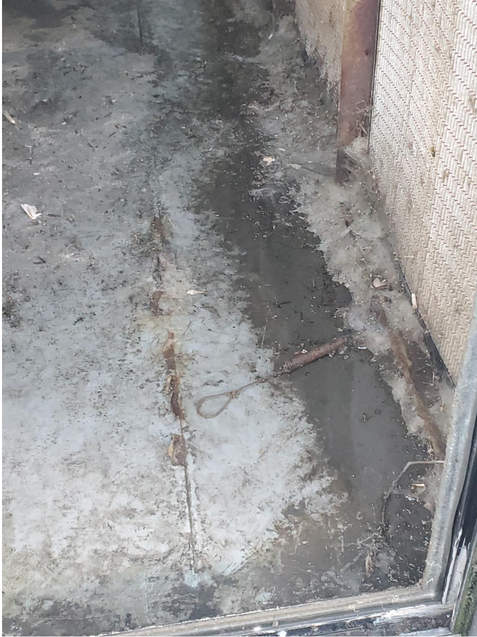
Photo 1: AHU-1 Outside Air Intake Plenum
