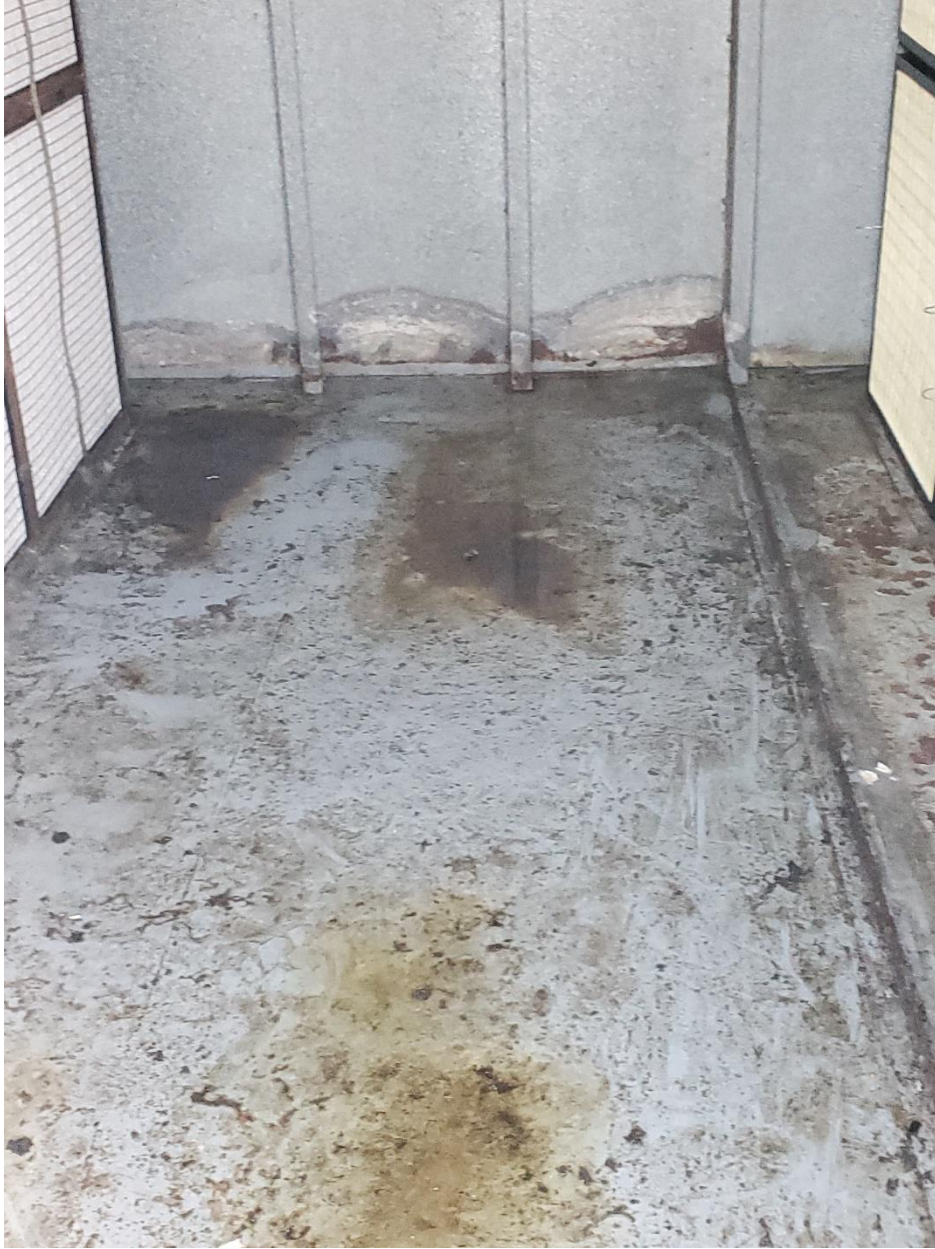
Photo 2: AHU-1 Filter Plenum
