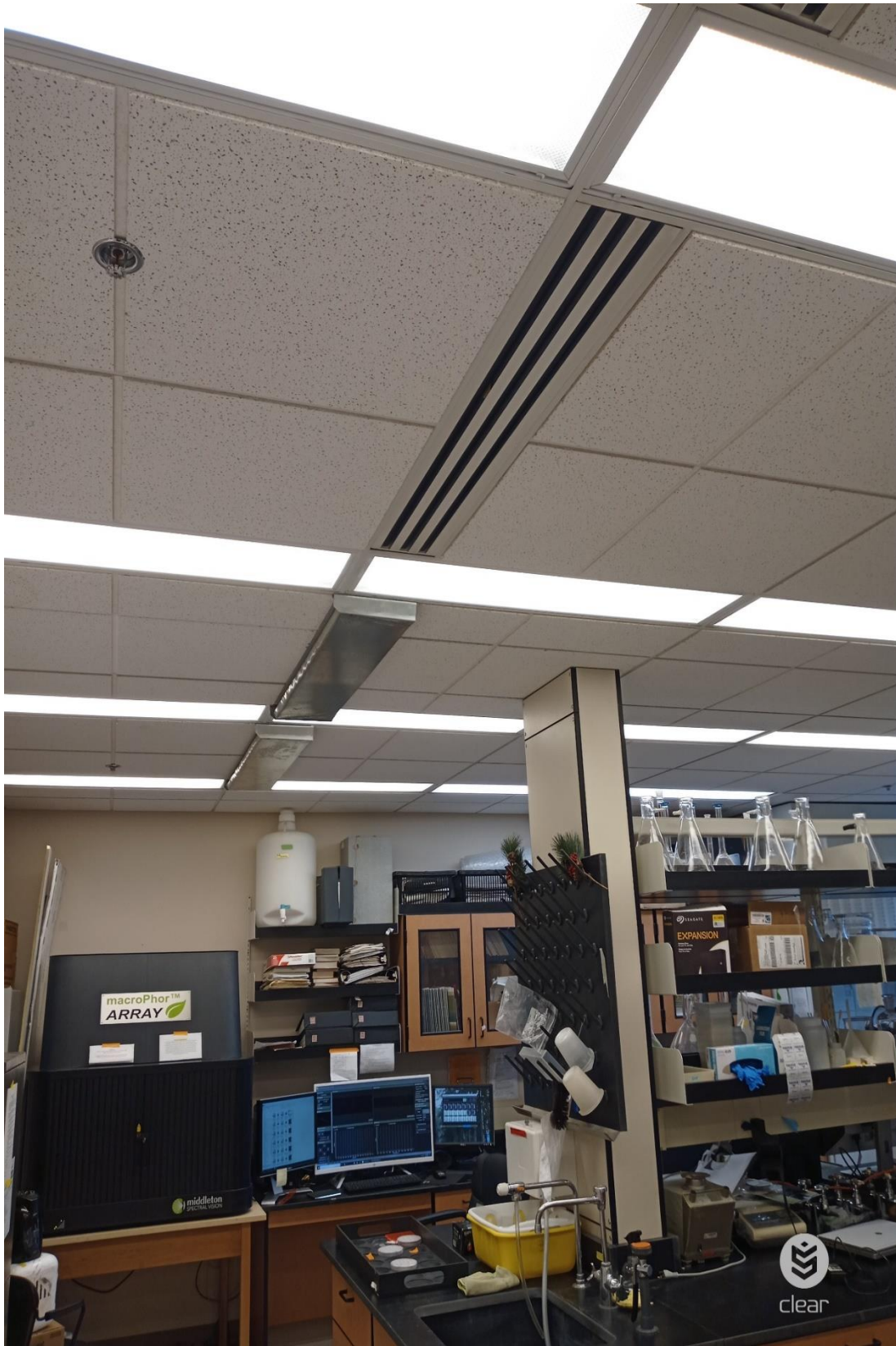
Photo 5: Linear Slot Diffusers in Laboratories
