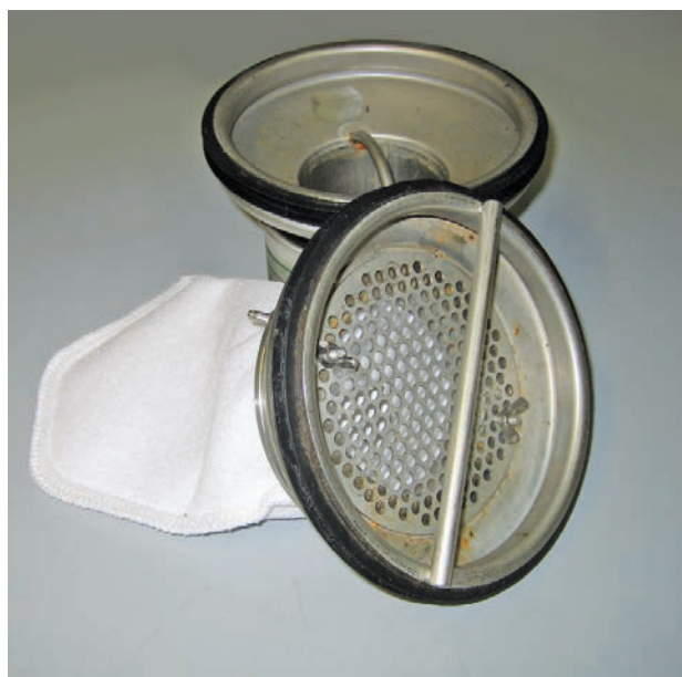
FIGURE 11. Filter Sock on Floor Drain*
