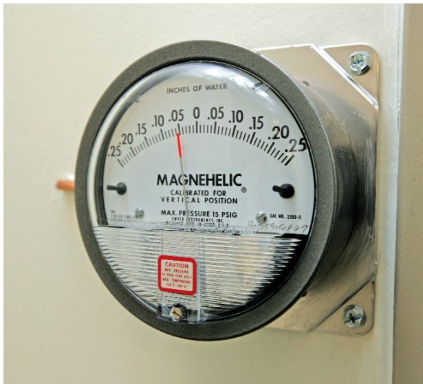
FIGURE 16. Magnehelic Gauge for Visual Confirmation of Pressurization
