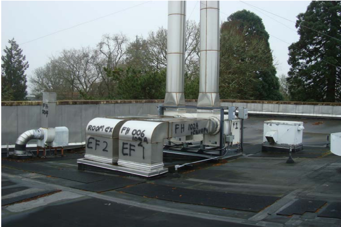
Roof Area "B" new equipment has been added.
