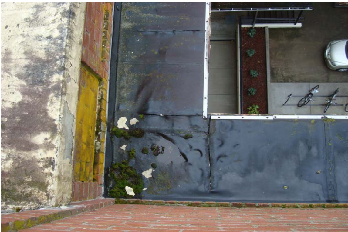
Roof Area "I" Cornice, Membrane failure typical.
