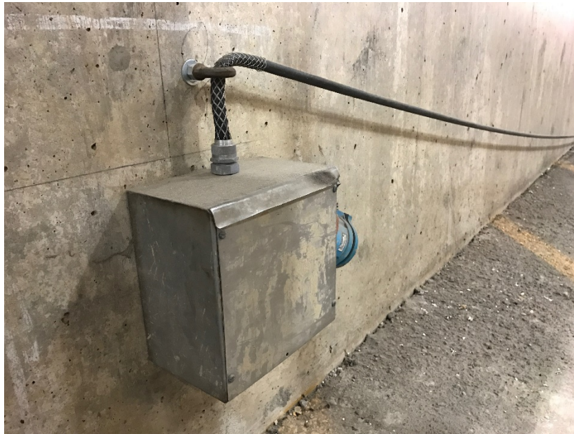
Figure 5. 480V/3 phase plugs located along the side of the flume.
