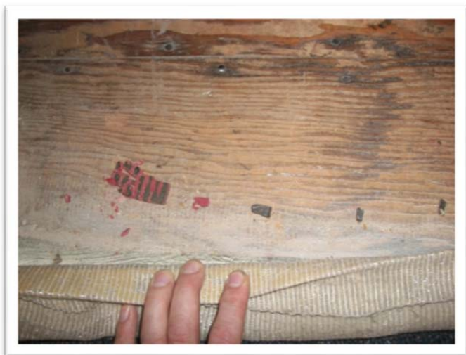
Assumed Asbestos Floor Tile, Room 314E Threshold
