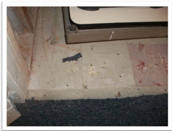
Sample 14-072A.12, 9" Floor Tile, ACM
