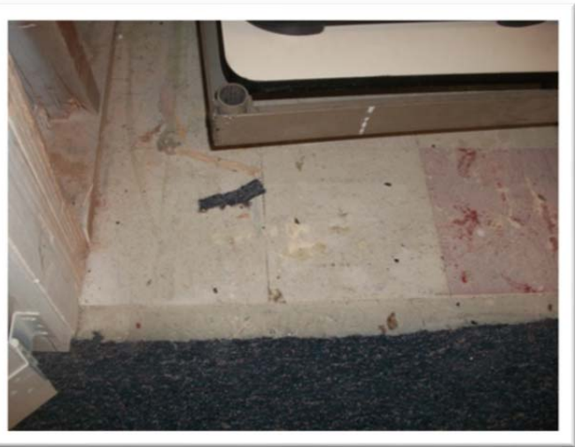
Sample 14-072A.12, 9" Floor Tile, ACM
