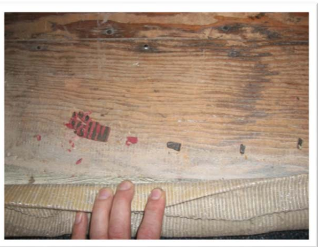
Assumed Asbestos Floor Tile, Room 314E Threshold
