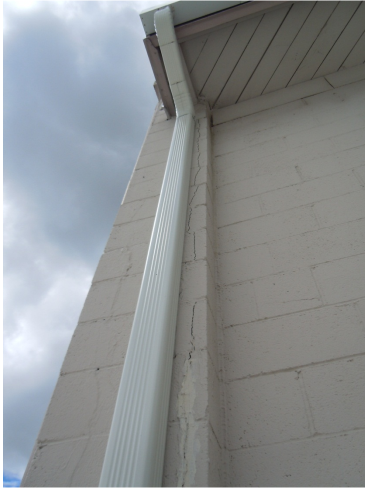
Figure 3.6 – Vertical Cracks at Southeast Corner of Gymnasium
