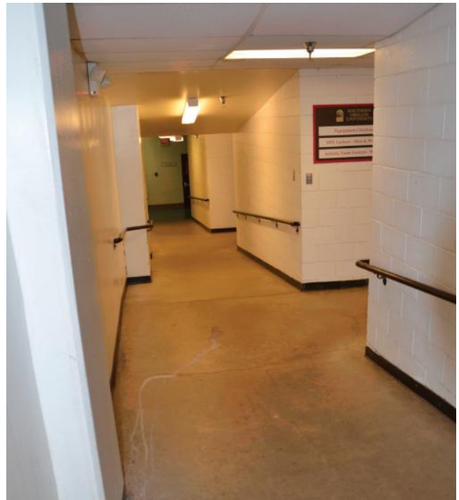
Non-compliant ramps, McNeal Basement
