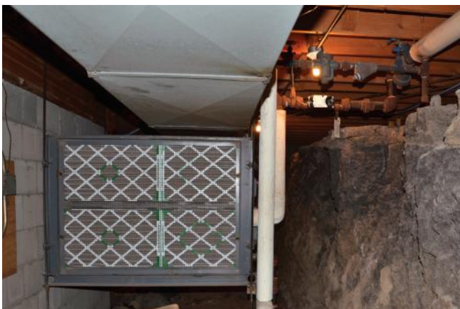
Air filters next to unexcavated basement
