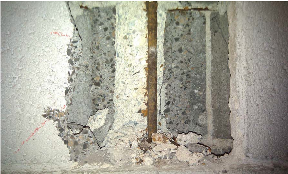
Figure 2: Corroded Steel within Wall
