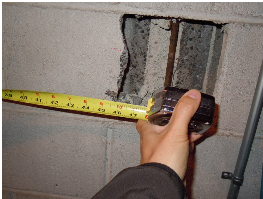
Figure 3.5 – Vertical Cracks Spaced at Four Feet
