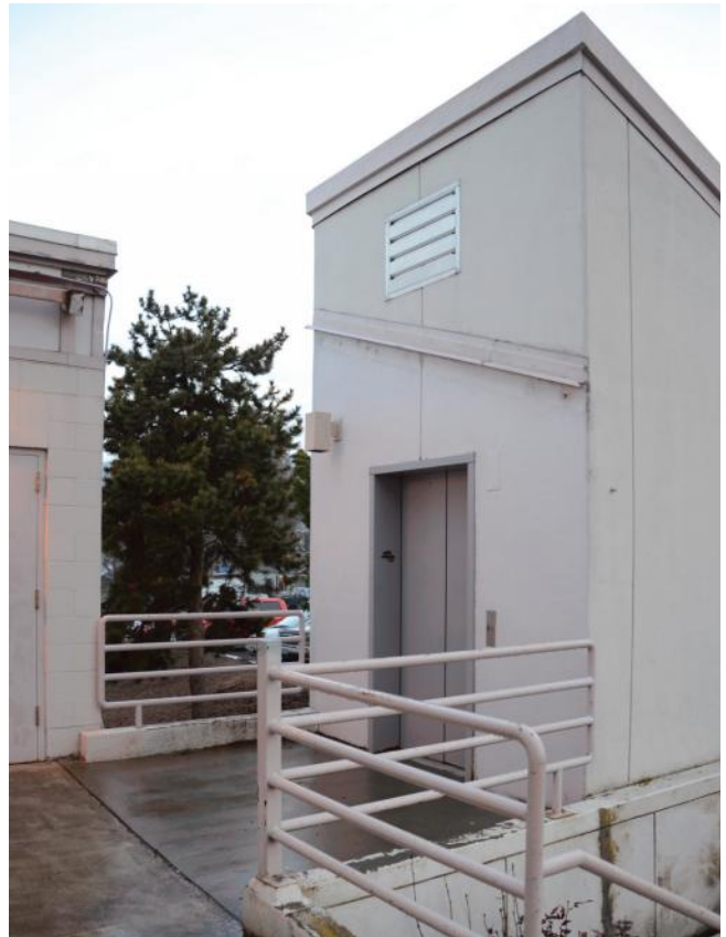
Outdoor & uncovered elevator
