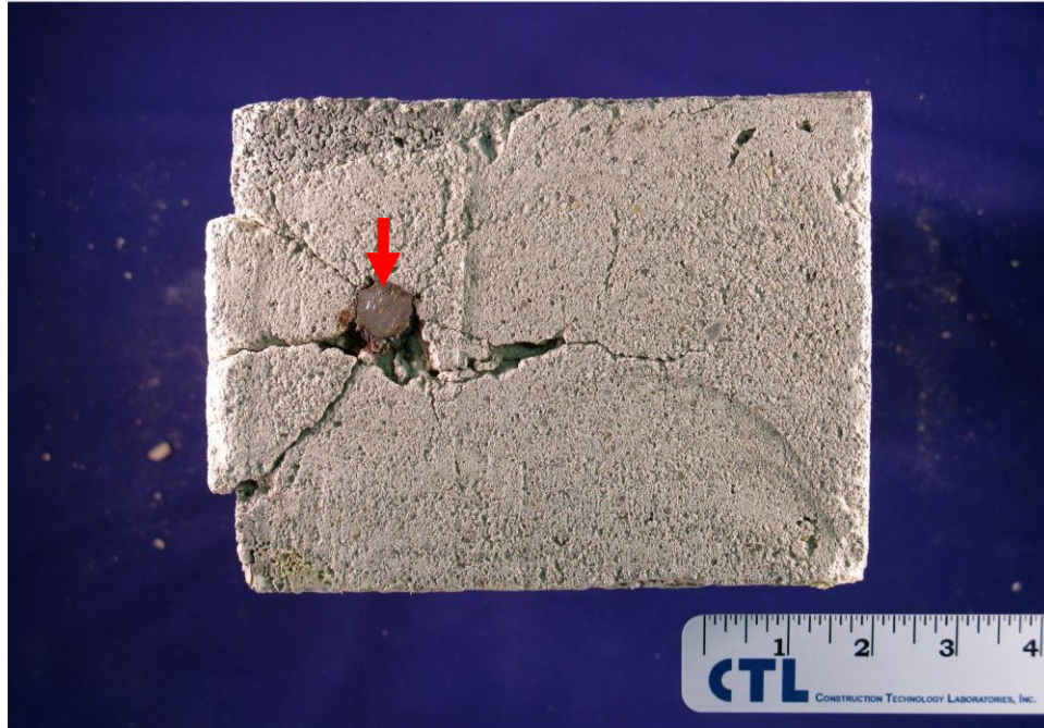
1c. Top surface showing cracks extending radially from a corroded reinforcing bar (arrow). The surface is covered with joint mortar.
