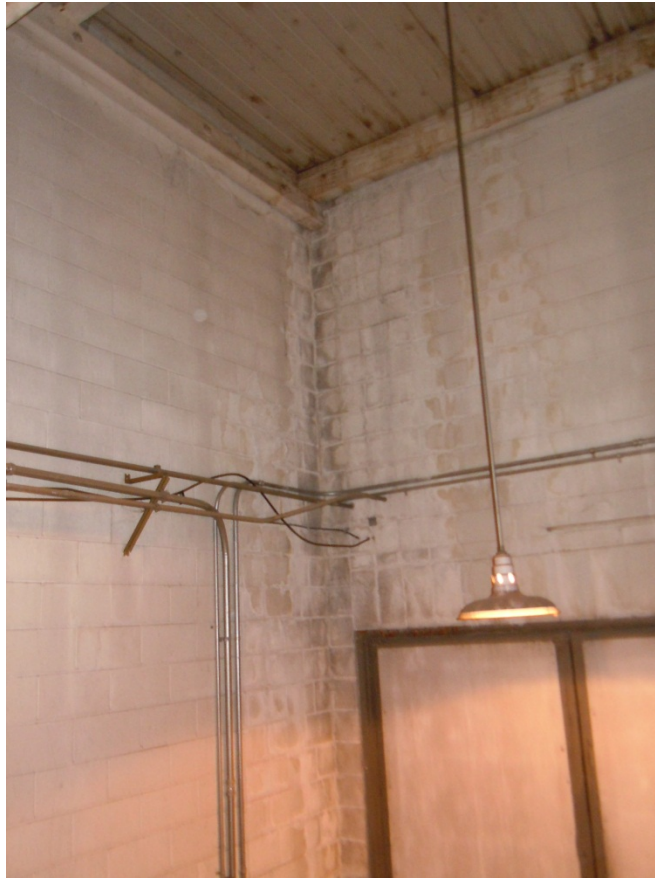
Figure 3.17 – Missing Pilaster in Boiler Room
