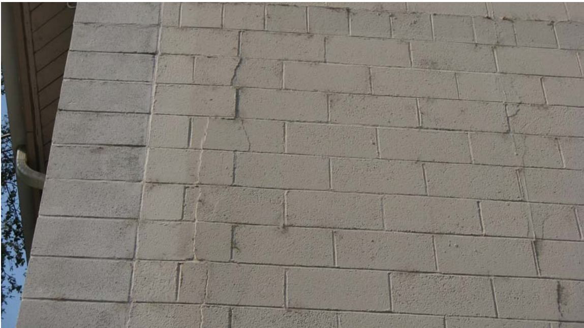
Figure 1: South West Wall Exterior Damage
