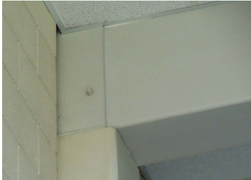
Figure 3.20 – Missing Nut in Pool Area
