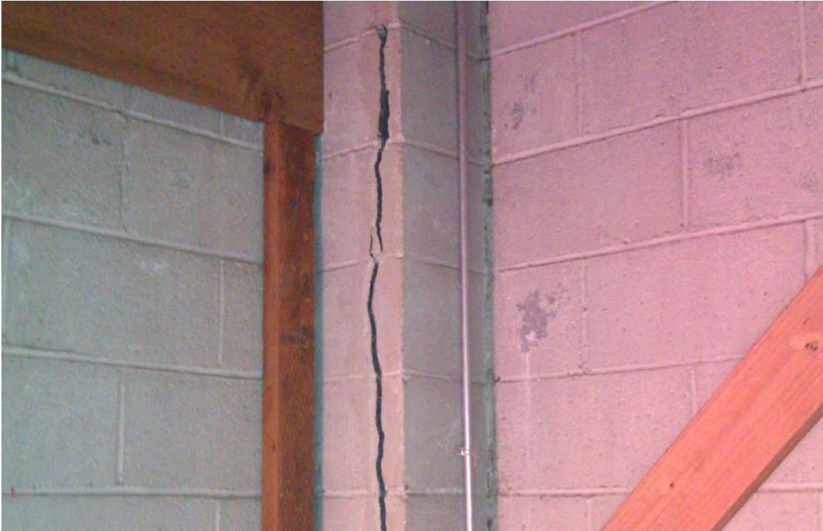
Figure 3: South West Wall Damage at Pilaster
