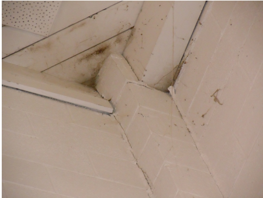
Figure 3.12 – Moisture at Top of Southeast Column
