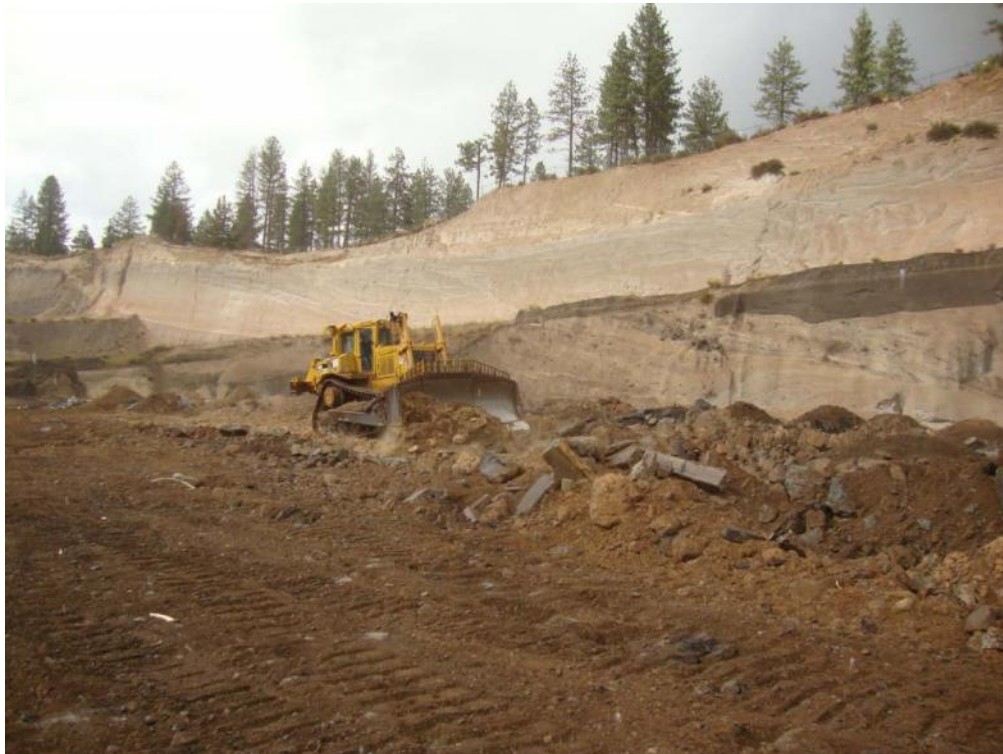
PHOTO 12: View of current backfilling and leveling activities being conducted in the eastern portion of the pit.
