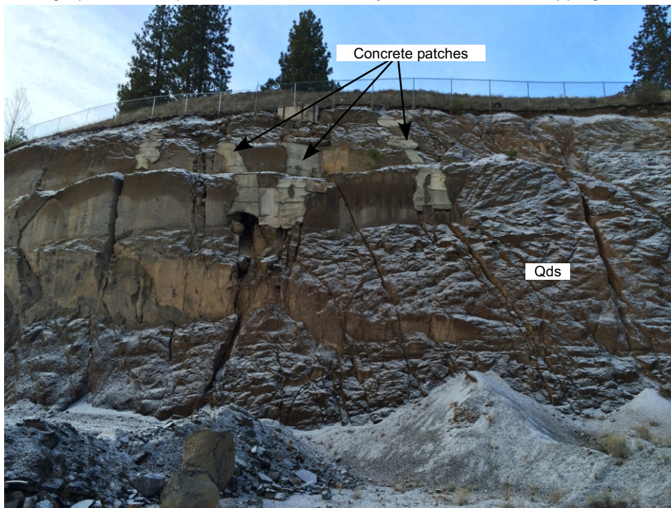
Photograph 4: Example of open joints and concrete patches in unit Qds.
