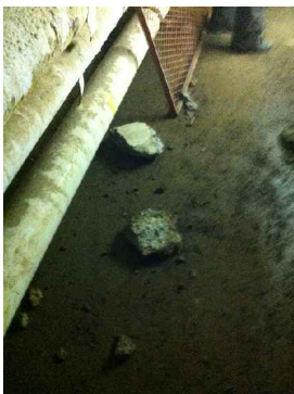
4 SPALLED CONCRETE ON FLOOR
