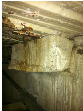
4 AT BLD'G FOOTING ( \pm 125' S OF ENTRANCE)
