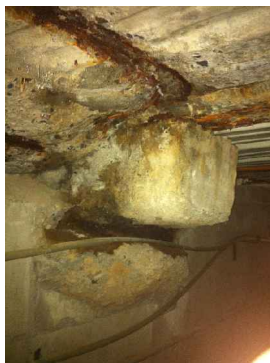
4 AT BLD'G FOOTING ( \pm 155' S OF ENTRANCE)
