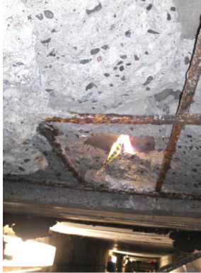
2 LID FAILURE IN TUNNEL
