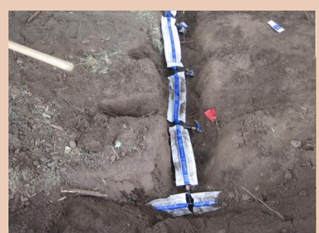
Figure 2.2.3: Hand trenching is used when a site is irregularly shaped or contains several obstructions.
