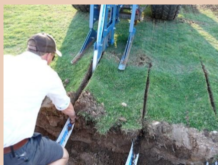
Figure 2.2.2: With the KISSS Plow, a crew can complete large areas quickly and with high consistency in depth and spacing.
