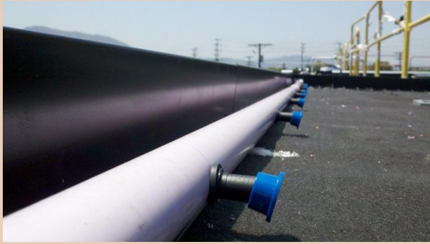
Figure 5.3.2: KISSS BFF Straight Ring-Lock Start Connectors protruding from the side of a Header pipe.
