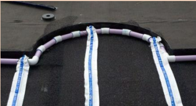
Supply Lines (Headers) and Flush Lines (Footers) See Section 4
