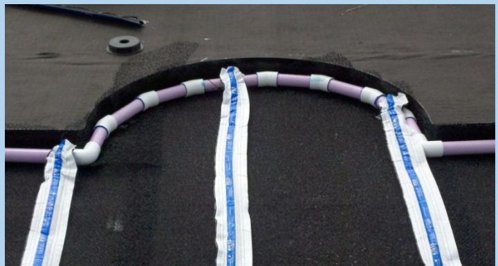
Figure 4.1.2: A footer pipe incorporating jointed pieces. Curved headers may be medium density MDPE.
