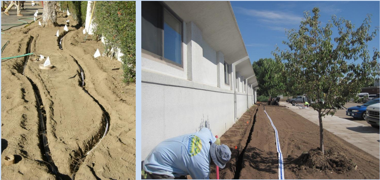
Figure 8.3.1: Hand trenching is the best installation method when in small or irregularly shaped plots
