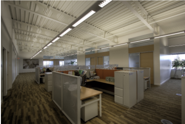
ABOVE view of exposed SMARTBEAMS installed at the Les Shwab headquarters in Bend, Oregon.
