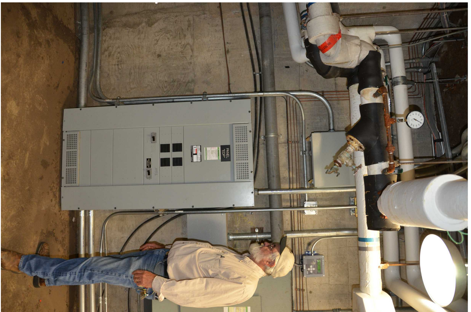
REPLACE EXISTING "EDP" WITH NEW 600A I-LINE "SDP" CONNECT EXISTING FIRE PUMP FEEDER TO FEED THRU LUGS.
