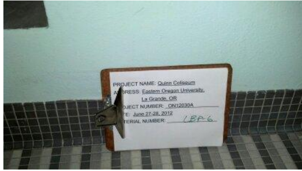
Photograph 14: Lead-containing paint (0.0022% lead) was identified in the paint sample LBP-6 obtained from the light blue wall paint located in the pool area.
