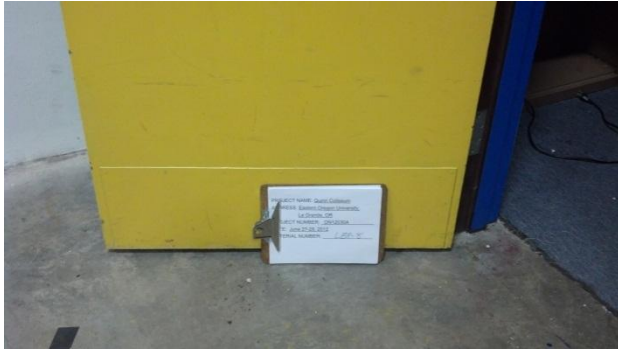
Photograph 10: Lead-based paint (1.0% lead) was identified in the paint sample LBP-8 obtained from yellow door paint located in the Balcony area over the gym.
