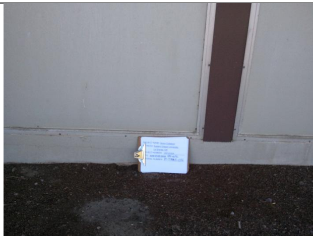
Photograph 16: The results of the PCB sampling activities indicated the window caulk sample M-CAULK-037-PCB contained 868 ppm PCB, which is above the 50 ppm EPA regulatory limit. This window caulk is associated with the transite panels on the north side of the building.
