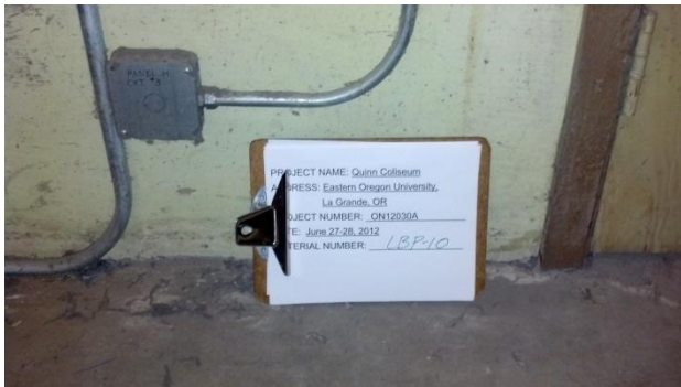
Photograph 12: Lead-based paint (0.63% lead) was identified in the paint sample LBP-10 obtained from the light green concrete wall paint located in the Janitor's closets throughout the building.
