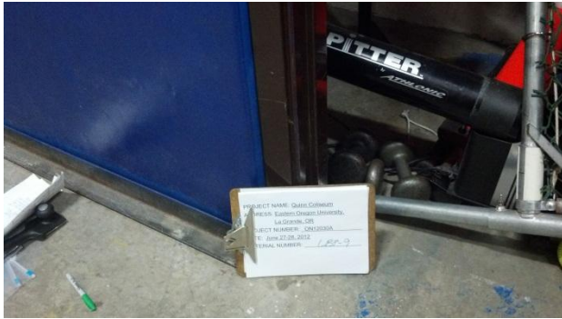
Photograph 11: Lead-based paint (3.6% lead) was identified in the paint sample LBP-9 obtained from brown door jamb paint located in the Balcony area over the gym.
