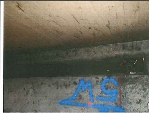
Fifth floor, west, note dry drain with standing water in gutter
