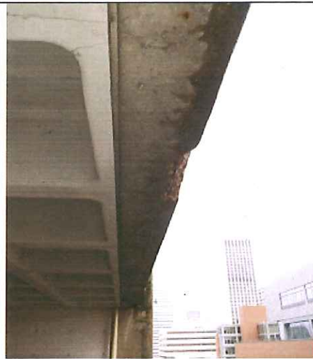
Eighth floor east elevation concrete beam deterioration
