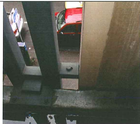
Fourth floor, west, standing water in gutter
