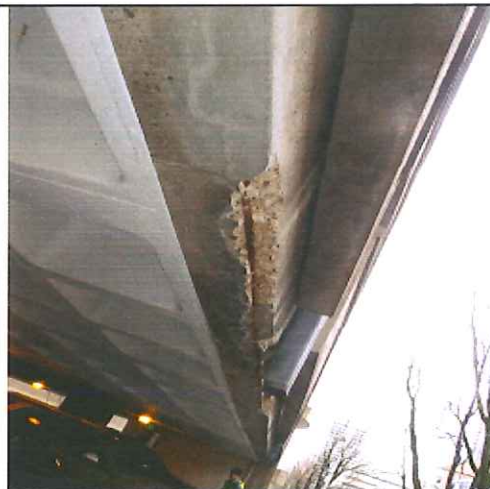
Third floor east elevation concrete beam deterioration.
