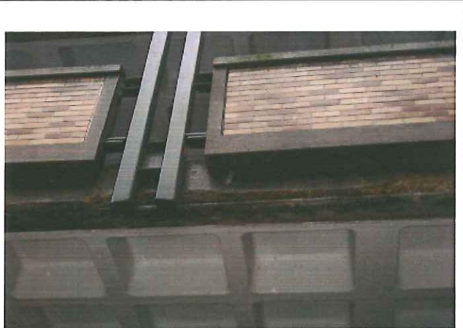
East Elevation, rebar is completely disengaged from the concrete beam.
