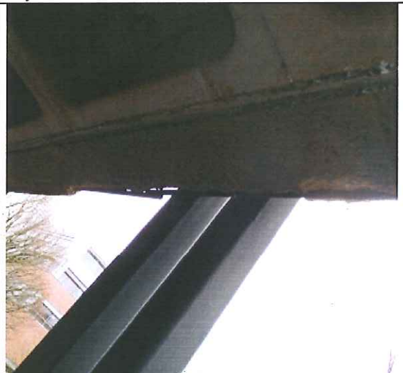
East Elevation, Fourth floor deterioration of concrete perimeter beam at T.S. connection
