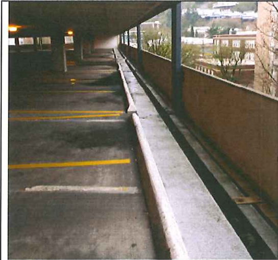
Seventh floor, west elevation, standing water at center of span and dry drains at each end.
