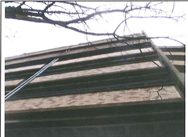
East Elevation, north end, similar conditions to the west elevation. The slope of the gutter in these areas is negative, causing water to overflow the gutter and run down the face of the panels.
