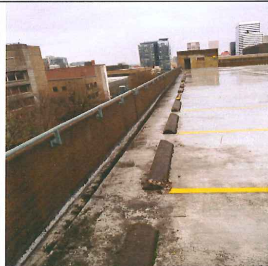
Eighth level, west guardrail, standing water at center while drains at ends are dry. Water is saturating the panel's cold joint and causing corrosion of steel reinforcement.
