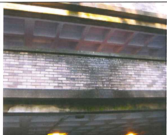
West elevation panel at level three, gutters at levels seven, six and five directly above do not drain. Water over flows the gutter at midspan while drains at each end remain dry. Heavy overflow conditions saturate the panels and edge beams below causing a buildup of moss and mildew and continuous deterioration of the steel reinforcement.
