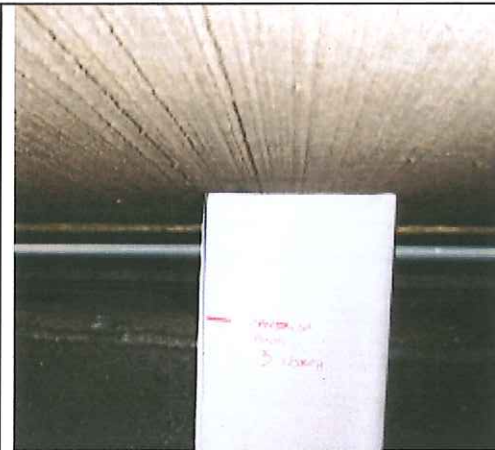
Typical panel 'bow' at center gap between panel and slab edge (1 1/2" to 2") Third floor north elevation center panel
