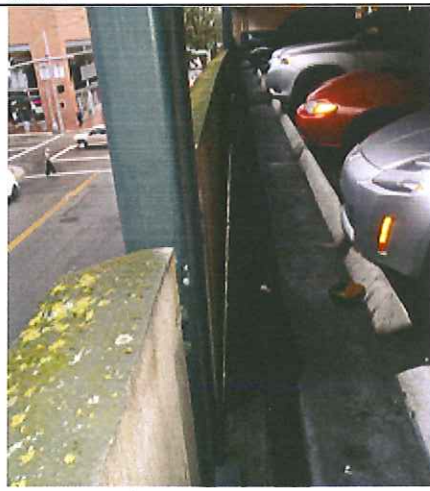
Third floor, north, standing water in gutter
