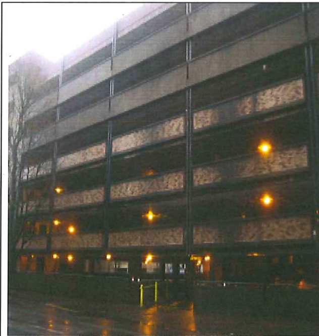
West elevation saturated by rain run-off and overflowing gutter system. Moss, mildew and general 'muck' coat several panels.
