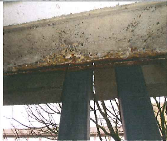
Sixth floor west elevation concrete beam deterioration
