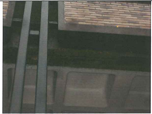
West elevation level 3, deteriorated concrete at beam at tube section connection.
