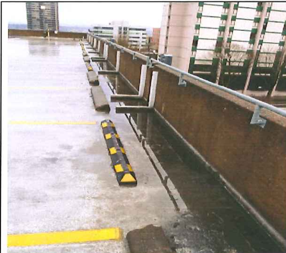
Eighth level, south guardrail, standing water at center while drains at ends are dry. Water is saturating the panel's cold joint and causing corrosion of steel reinforcement.
