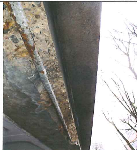
Third floor east elevation concrete beam deterioration.
