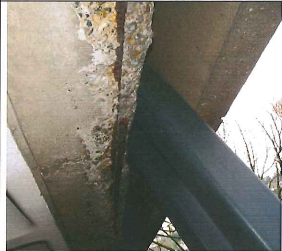
Sixth floor west elevation concrete beam deterioration
