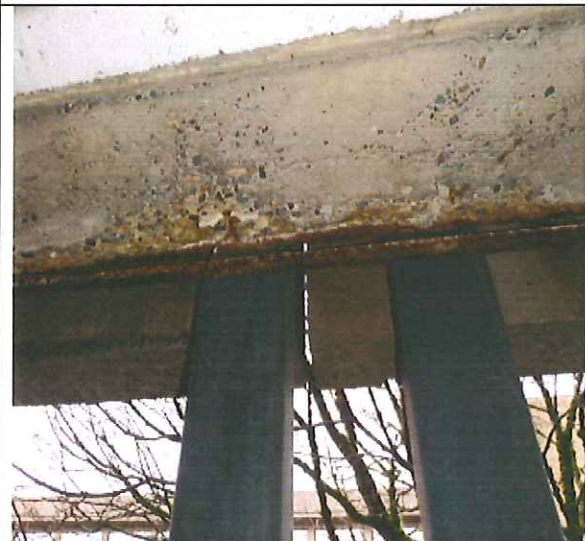
West Elevation, Fifth floor deterioration of concrete perimeter beam at T.S. connection
