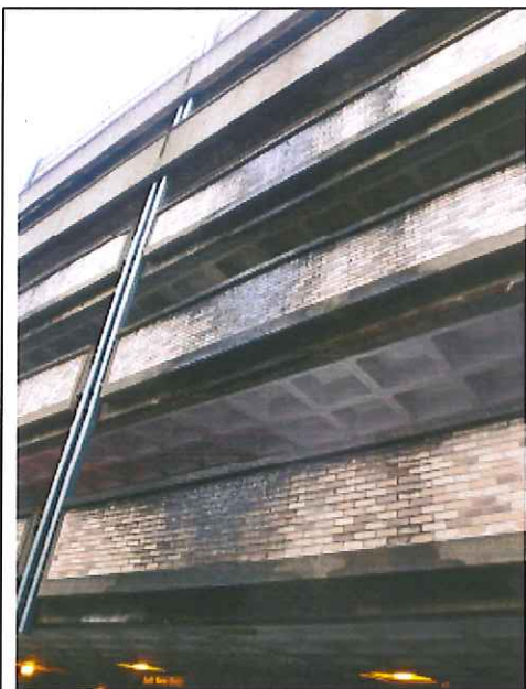
West elevation, center panels, moss, mildew growth on panels due to water running down the face and saturating the panels.
