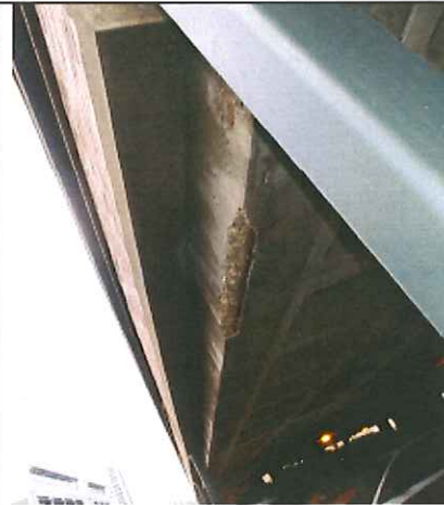
Fifth floor north elevation concrete beam deterioration.
