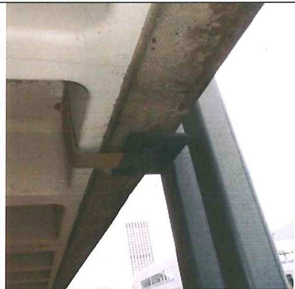
East Elevation eighth level slab /T.S. connection, note repair plate installed and water stained saturated concrete beam.
