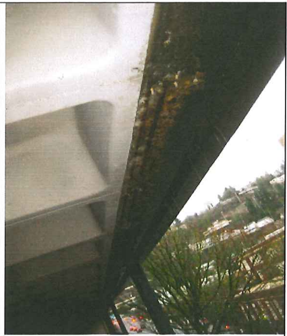
West elevation saturated by rain run-off and overflowing gutter system. Fifth floor looking up at sixth floor perimeter concrete beam.
