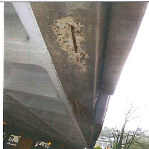
Third floor west elevation concrete beam deterioration.
