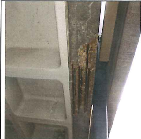
Seventh floor north elevation concrete beam deterioration
