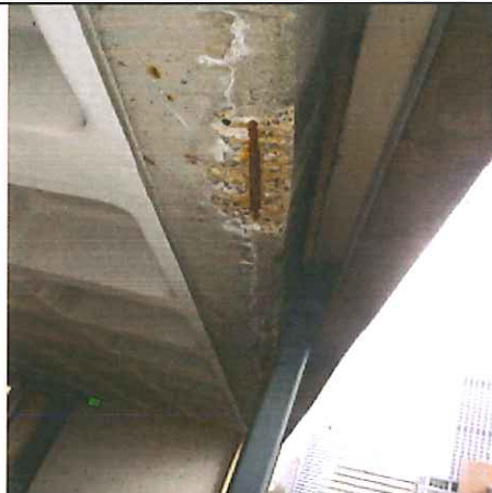
Seventh floor east elevation concrete beam deterioration
