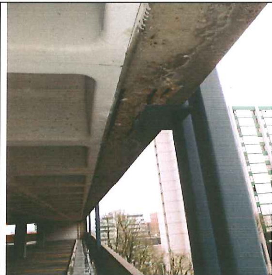
South Elevation eighth level slab /T.S. connection, note extensive deterioration of concrete beam at this location.
