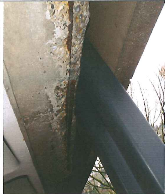
Deterioration of the perimeter beam occurs at or near many of the T.S. connections.
