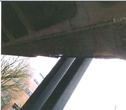
Fifth floor east elevation concrete beam deterioration.
