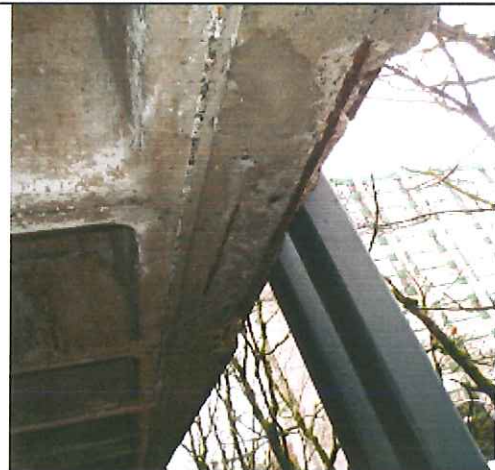
Fifth floor west elevation concrete beam deterioration.
