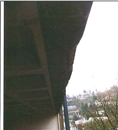
Eighth floor west elevation concrete beam deterioration
