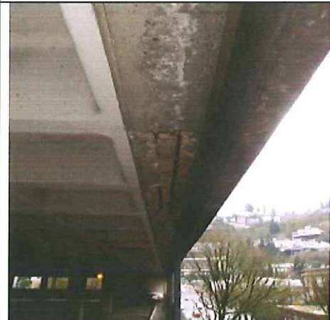
Seventh floor west elevation concrete beam deterioration
