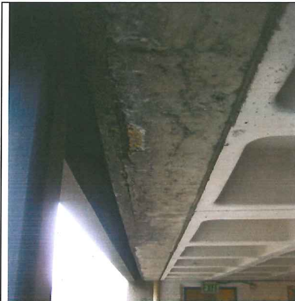
West elevation perimeter beam deterioration at steel tube section connection.
