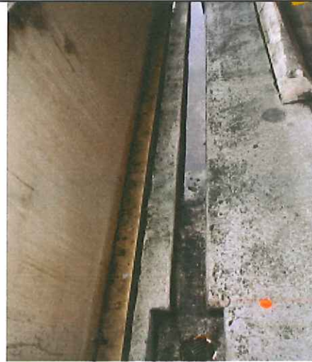
Seventh floor, west elevation, south end of gutter.
