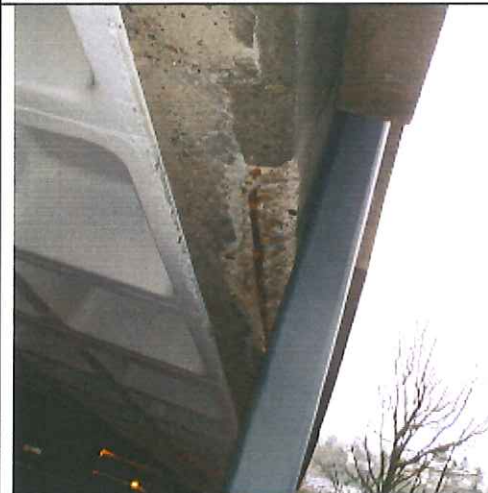
Fourth floor west elevation concrete beam deterioration.
