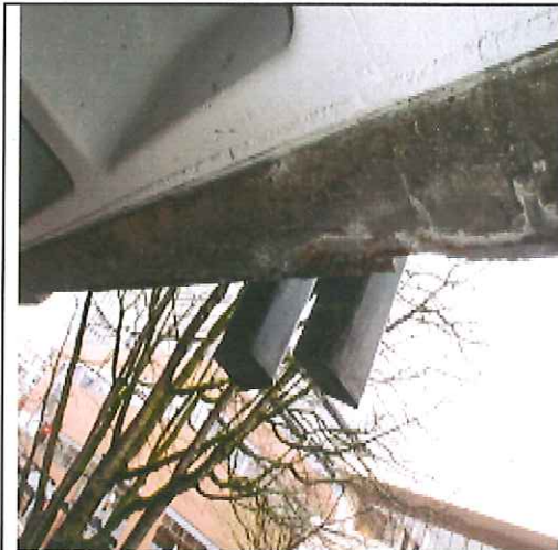
Third floor east elevation concrete beam deterioration.
