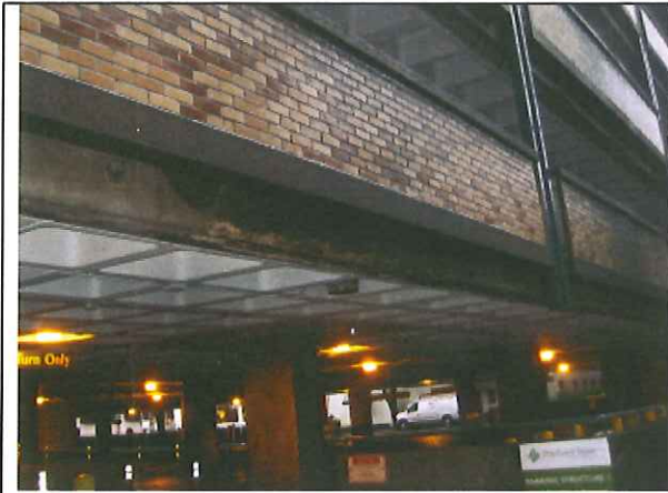
West entry, deteriorated concrete at beam
