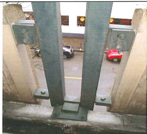
Typical Panel connection, note slotted holes at top connect opposite from bottom connection. Panel cannot move at this connection
