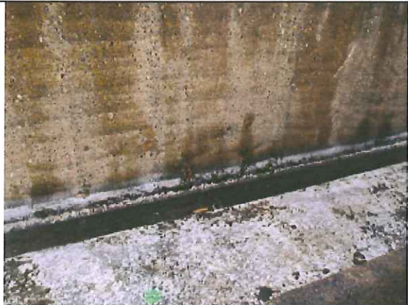
Eighth level, north guardrail, exposed panel reinforcement and deteriorated water proofing at cold joint
