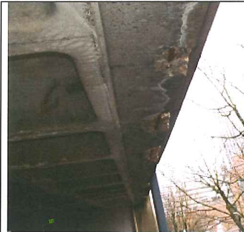
Fifth floor east elevation concrete beam deterioration.
