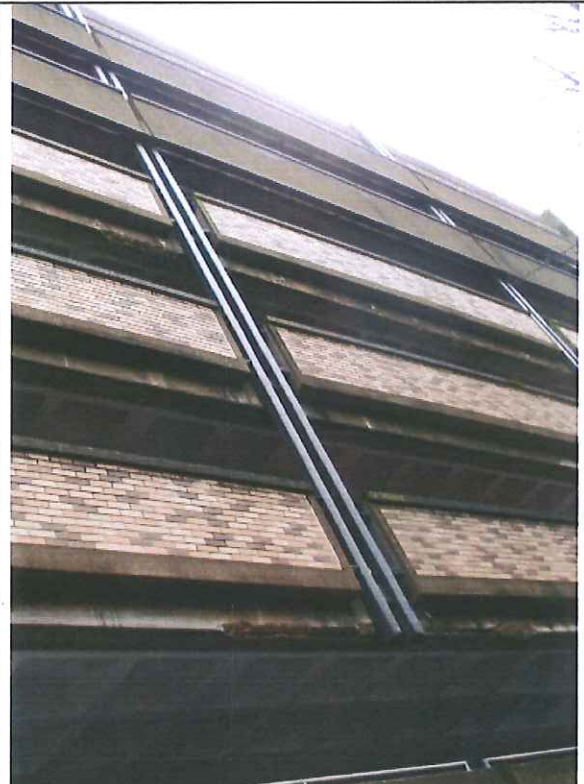
East elevation , deterioration at or immediately adjacent to the tube section connections
