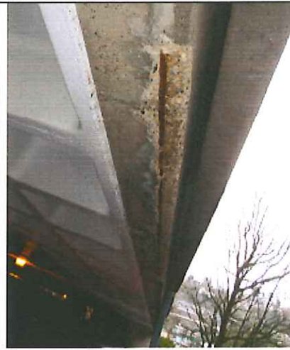
Fourth floor west elevation concrete beam deterioration.
