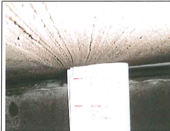
Typical panel /slab edge gap at end connection (1/2" +/-) Third floor north elevation center panel
