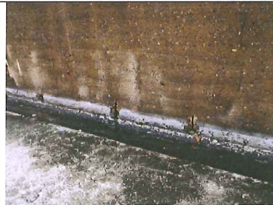
Eighth level, east guardrail, exposed panel reinforcement and deteriorated water proofing at cold joint
