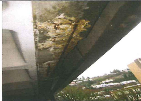
West Elevation, rebar is completely disengaged from the concrete beam.
