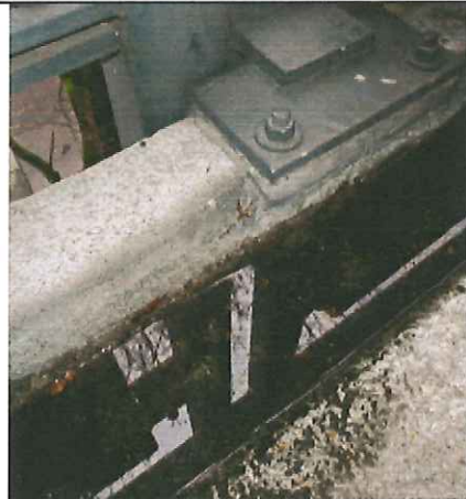
Fifth floor, west elevation, standing water in drain
