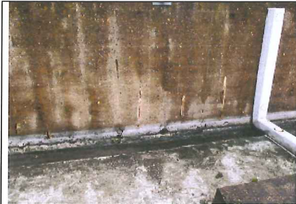
Eighth level, south guardrail, exposed panel reinforcement and deteriorated water proofing at cold joint
