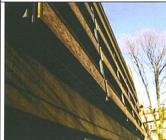
South Elevation, bowed panels. Some panels bow out as much as 2" in the center
