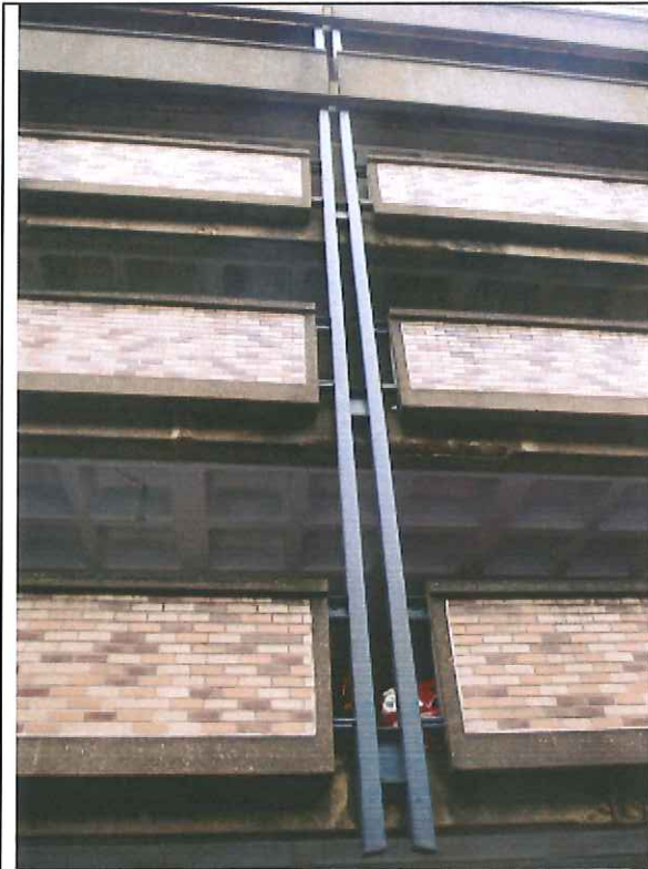
West elevation , deterioration at or immediately adjacent to the tube section connections
