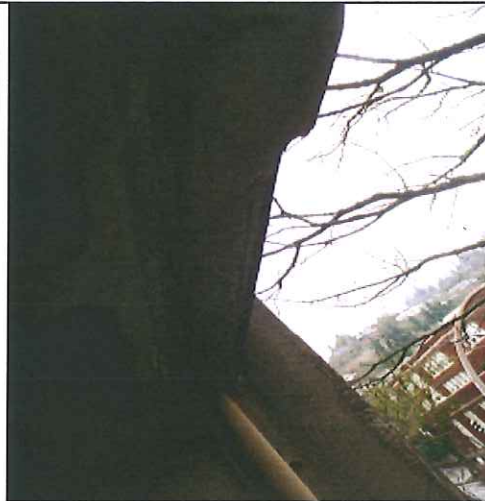
Fifth floor west elevation concrete beam deterioration.
